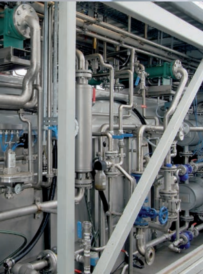
A complex system of pipes with an integrated heat exchanger
